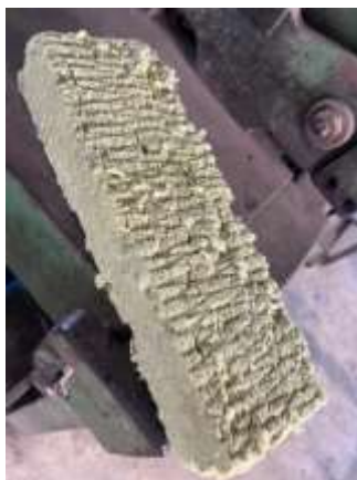
Fig. 4. Refractory fiber lining.
